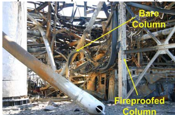
Figure 8 – Collapse of Non-Fire Proofed Structural Steel
