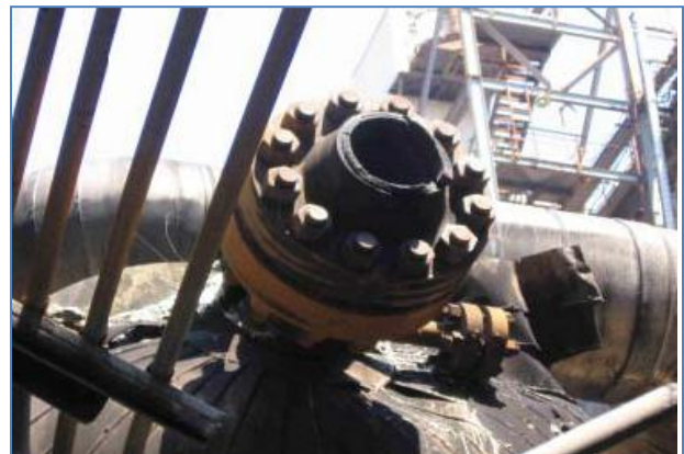
Figure 10 – 8” NPS Hydrogen Piping Severed
