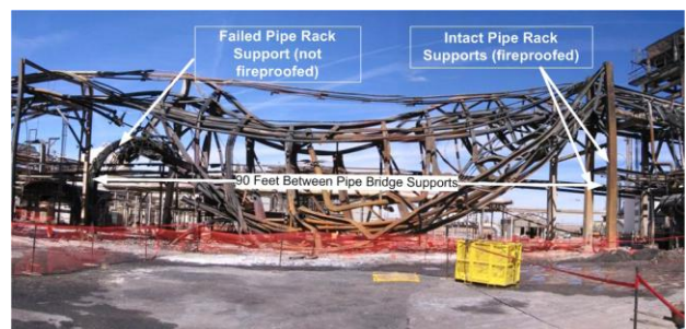
Figure 4 – Collapsed Pipe Rack as a Result of Heat from a Jet Flame.
